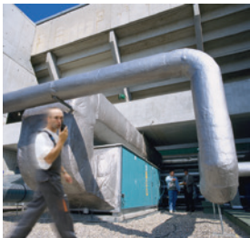
Air handling unit
