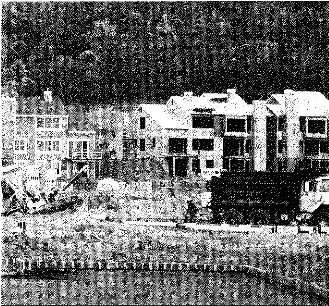
Construction sites requiring temporary power supplies can benefit from the ease of installation and portability of the Mini Power-Zone package power supply.
