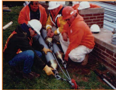
Tighten pulling eye so that it expands against interior of the conduit.
